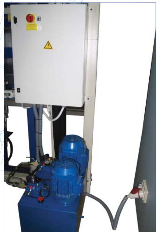
Figure 20. Electrical control panel.
